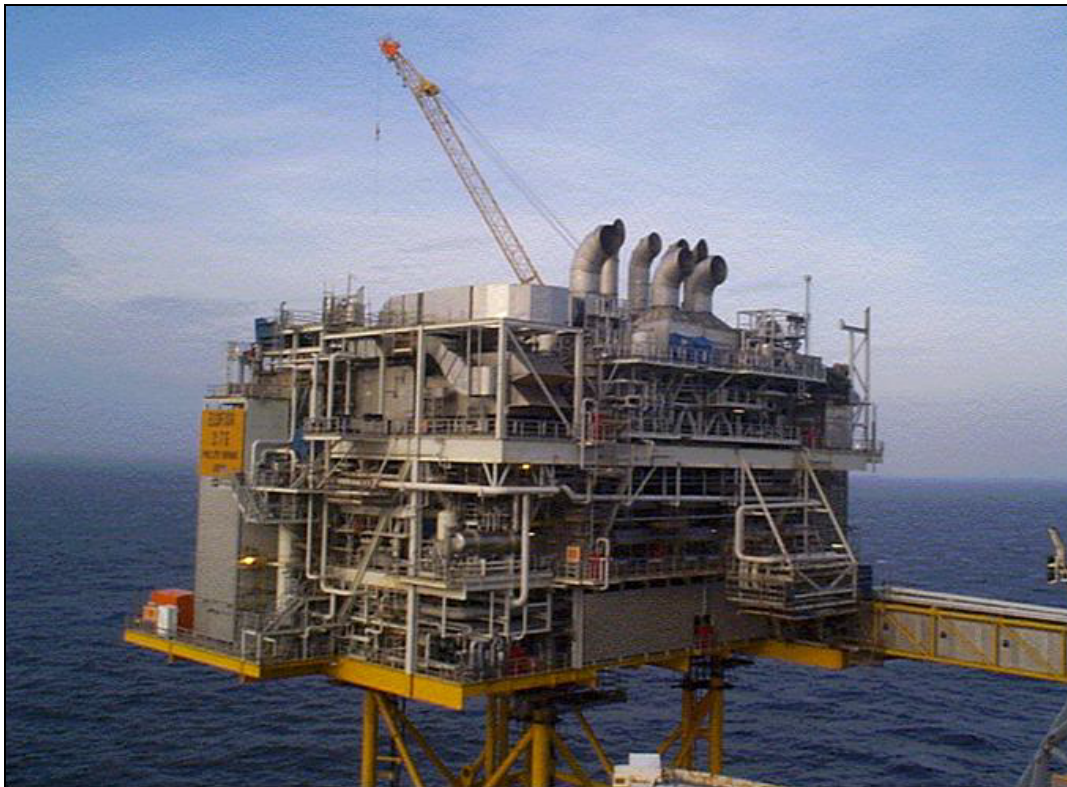
Figure 7.21: Example of a combined cycle power plant installed on an offshore platform on the Norwegian continental shelf [25, ABB, 2000]
